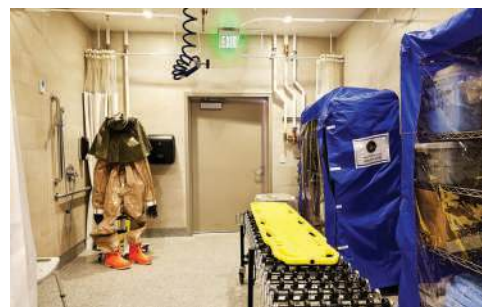
Contamination Patient Room at the new IHC Hospital ER
